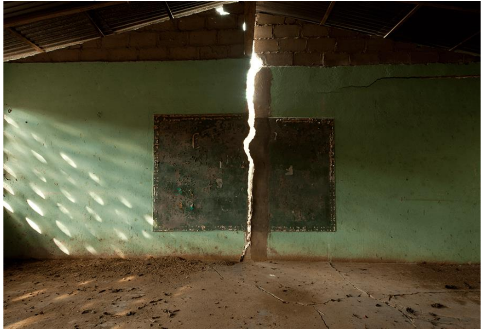
Figure 3. Silence with crack , Las Palmas, Bolívar, Colombia
